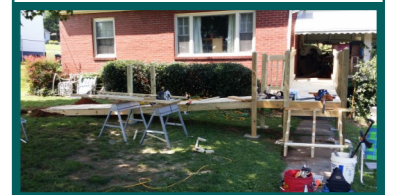
IOA partners with Lynchburg Baptist Association's Kingdom Builders to install ramps for needy families.
